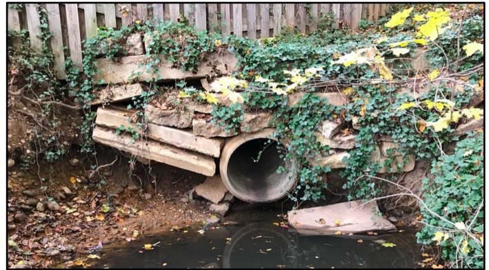
Map of the project and photo of the damaged pipe
